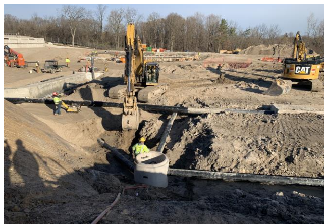
Photo 4: Final Clarifier 12" Drain Piping and Manhole
