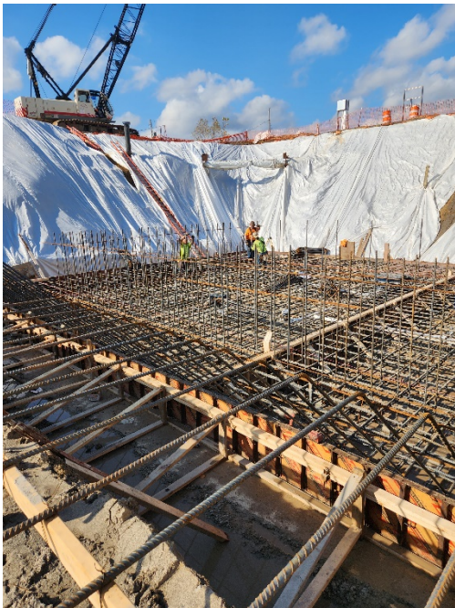
Photo 3: Placement of Top Mat of Rebar and wall dowels for the Dry Pit area of the EQ Basin.
