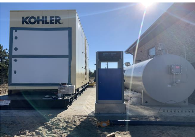
Photo 5: Electrical Building Generator and Fuel Tank
