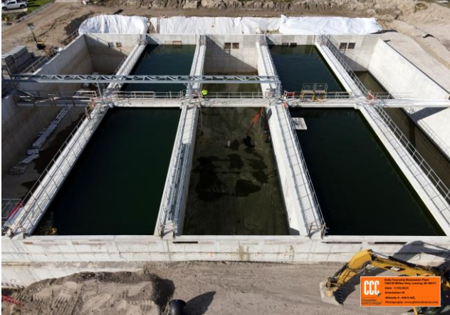
Photo 1: Aeration Tank Overview
