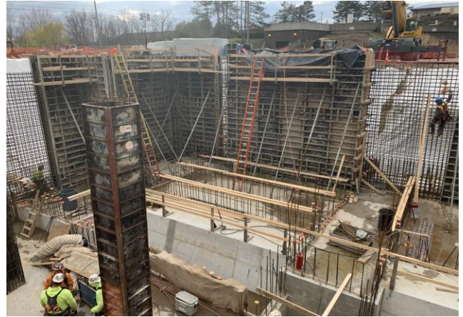
Photo 8: Headworks Building Interior Overview
