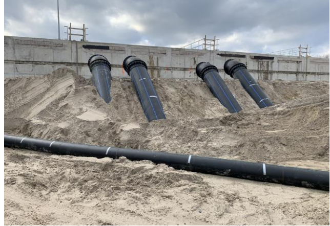
Photo 2: Aeration Tank 36" ML Piping
