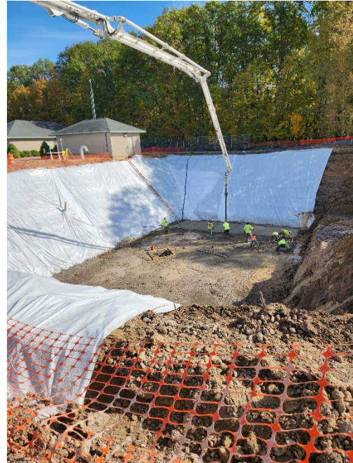
Photo 2: Placement of Mud Mat for the Dry Pit area of the EQ basin.
