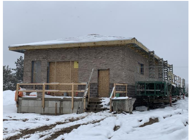
Photo 8: Electrical Building; brick and split face
