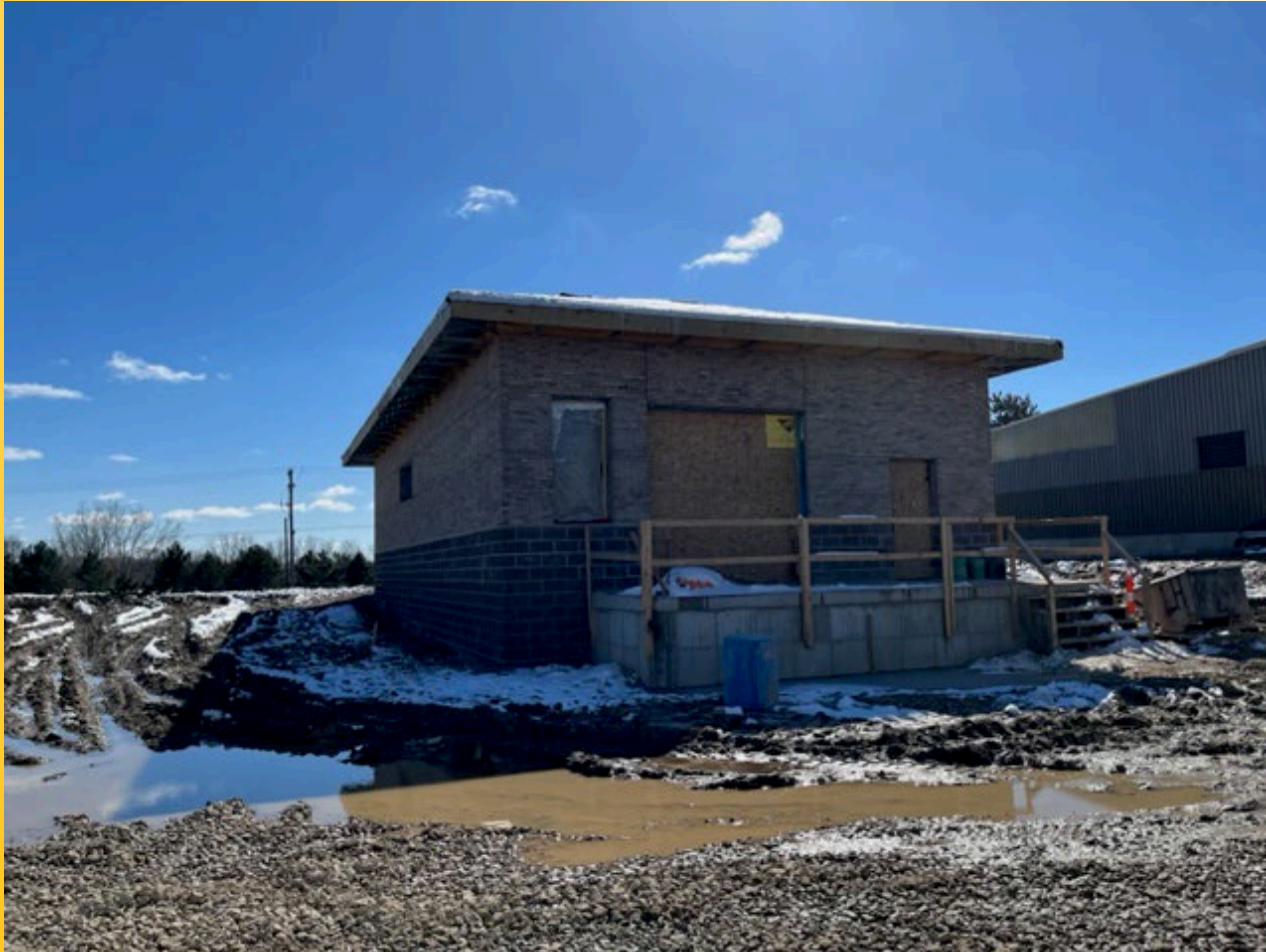
Electrical Switch Gear building
